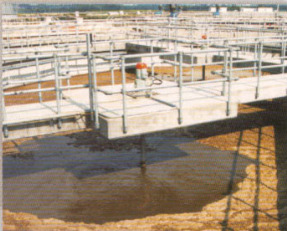
Biological Reactor Mixer
